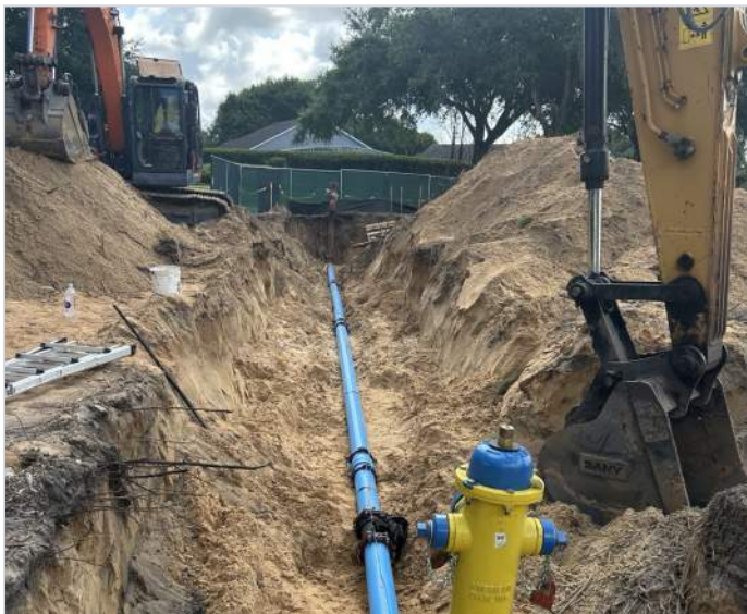
FIRE-WATER MAIN & HYDRANT
